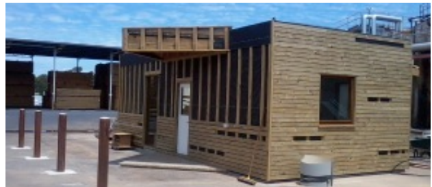
Figure 14: Horizontal timber cladding with Proctor Wrap Black Label building paper visible while under construction
