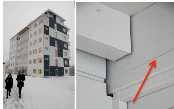
Figure 7: Splits evident in the CLT in the Älvsbacka Strand building by White Architects and built by Martinsons
