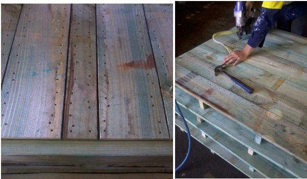
Figure 10: Detail of the nailing configuration and example of manufacturing the panels by hand.
