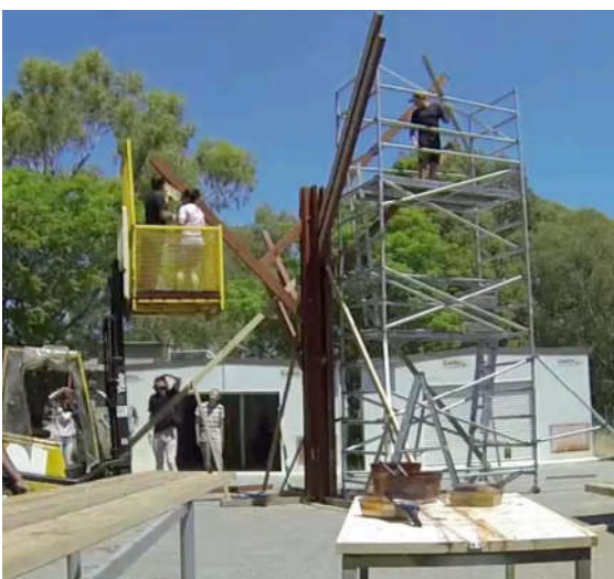
Figure 20: Central column and outriggers temporarily propped in place. Note the use of scaffold and caged safety platform.
