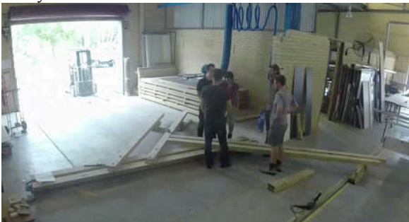
Figure 19: Half of the central column and outriggers being assembled on the workshop floor.
