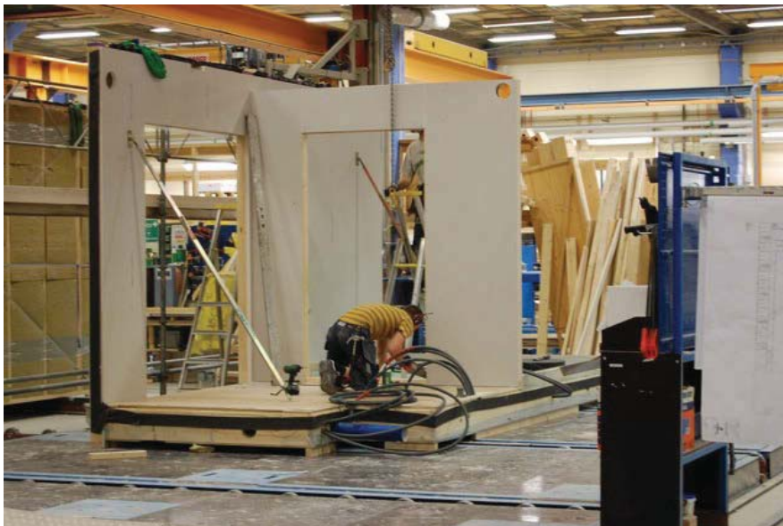
Figure 1.50 Lindbäck's Bygg's Lean factory floor layout showing the production flow and below, a tradesman working on a module. Flow diagram supplied by Lindbäck's Bygg. Photograph by D.Bylund
