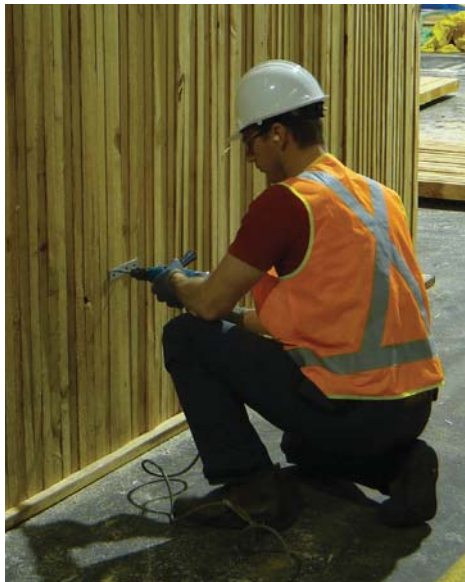
Figure 2.19 Fixing the 'H' acoustic wall tie to the external face of the outer GPLT leaf using an electric drill and a #2 Phillips head driver. Photo D.Bylund
