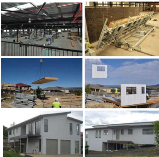
Figure 1.32 panelBuild manufacturing plant, on site installation and completed houses Information and images sourced from panelbuild.com.au and a factory visit by the author.
