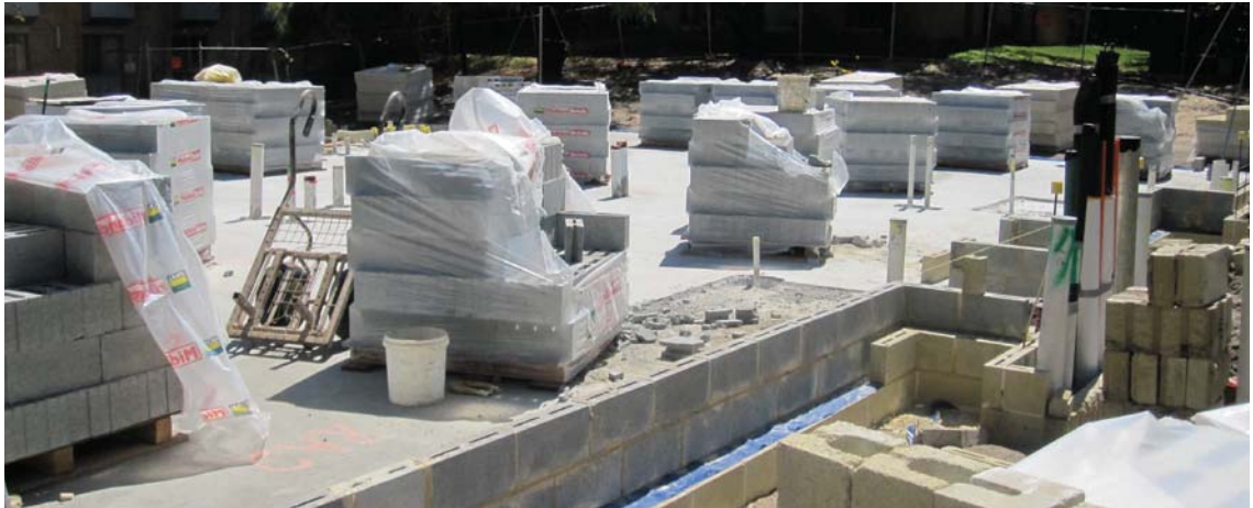
Figure 2.25 Brick packs delivered to the Currie Hall building site waiting to be laid. Image supplied by Palassis Architects
