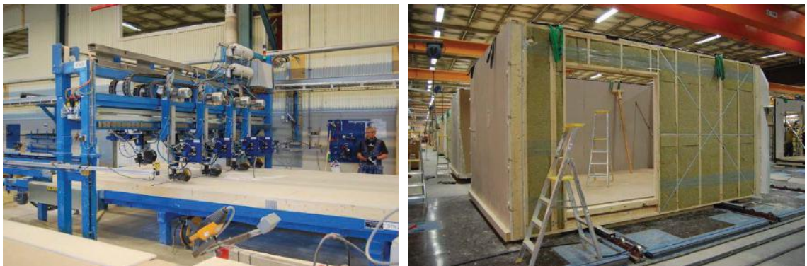
Figure 2.26 Lindbäcks' automated timber floor panels under construction and volume module production line in Sweden. Photo. D.Bylund
